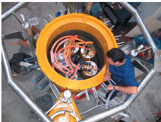
Fig. 2 - The fully assembled Junction Box during the filling of the fiberglass vessel with silicone oil.
