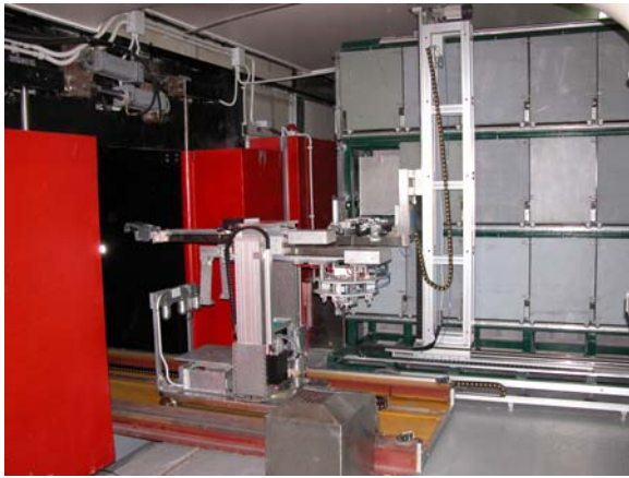
Figure 3 : remote handling system of the TIS.
