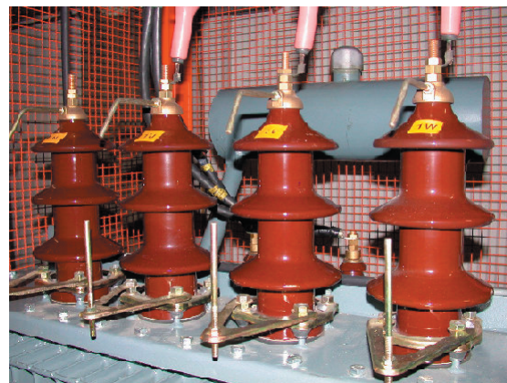
Figure 1: the new high voltage transformer already installed.
